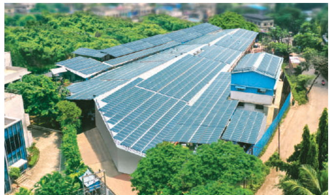
Massive State-of-the-art manufacturing facility with solar panels, in Vasai
